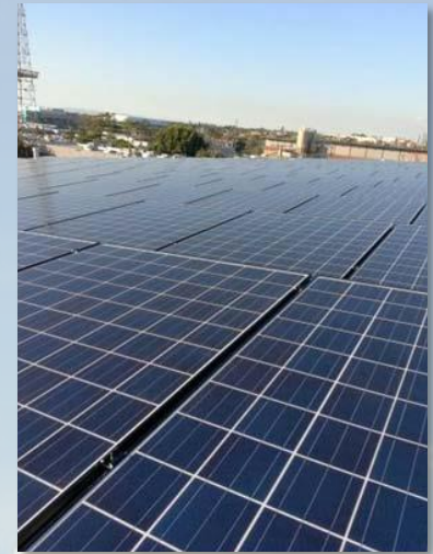
Signal Hill Facility
